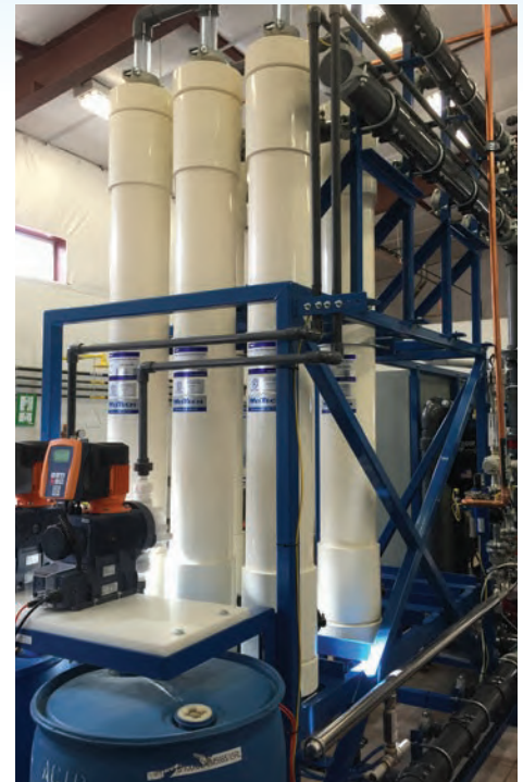
Only half the ultrafiltration racks are populated due to current demand. The capacity of the system can be doubled quickly and inexpensively by installing additional modules. All system components are sized for the increased capacity to limit costs associated with expanding the system.
