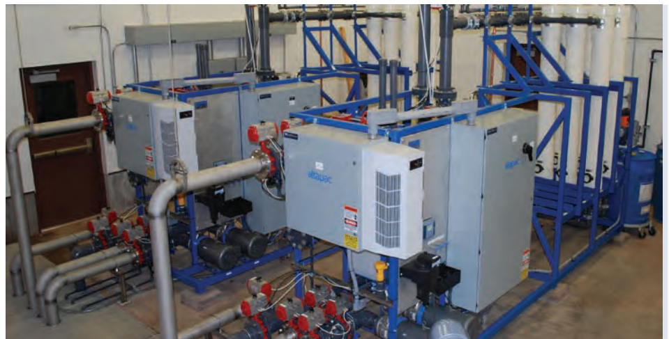
The compact and efficient design of the AltaPac limited the costs of installation and construction of the new treatment building.
