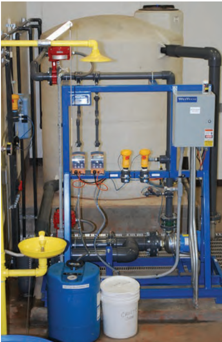
An optional neutralization system was included with this equipment to allow for discharge of chemical solutions used during membrane cleaning.
